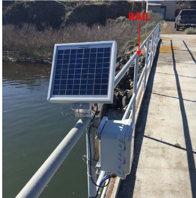
Figure 3. Water level data collection platform with RAIL point marked.
